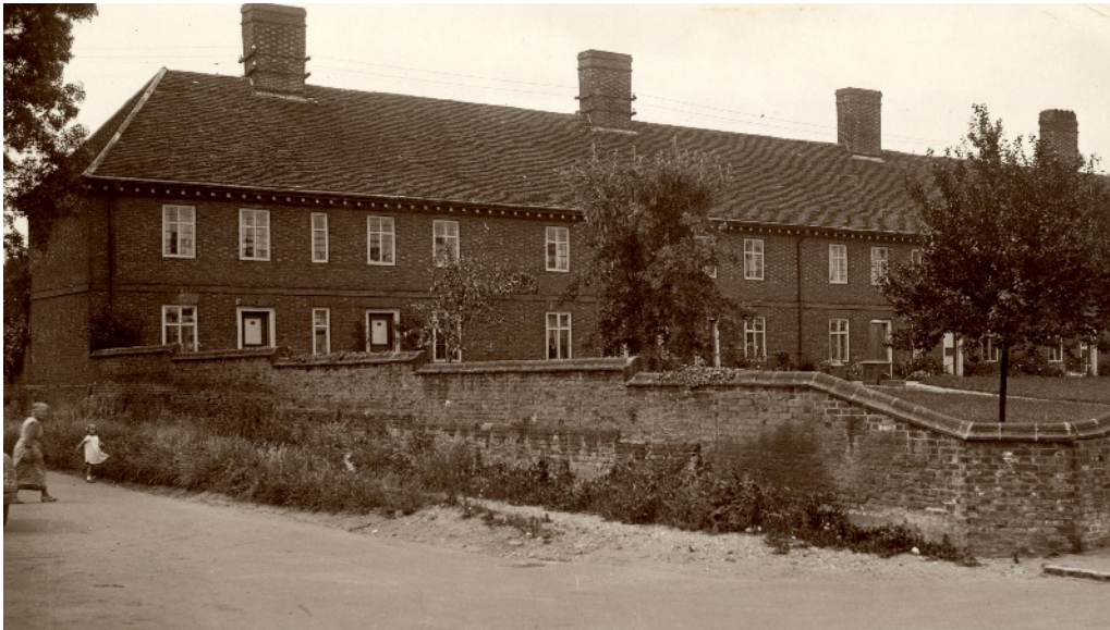
Electricity cables supported from chimneys on the Mills almshouses, Framlingham Author's collection
